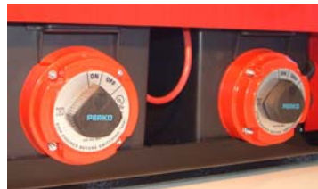
Main Safety Switch & Power Supply Switch
